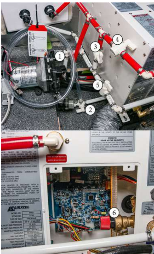
Figure 8.1 - water heater (located roadside under bench)
